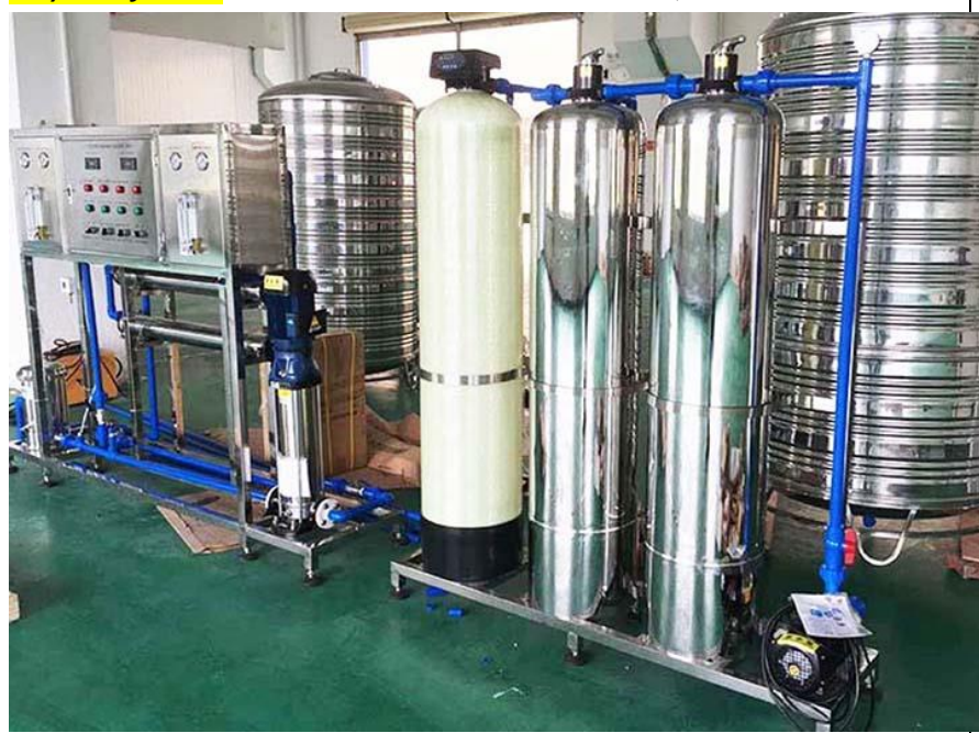
4.1) RO system: SUS304 Sand filter & carbon filter;
